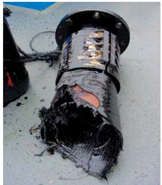
^ Failed bunker hose
