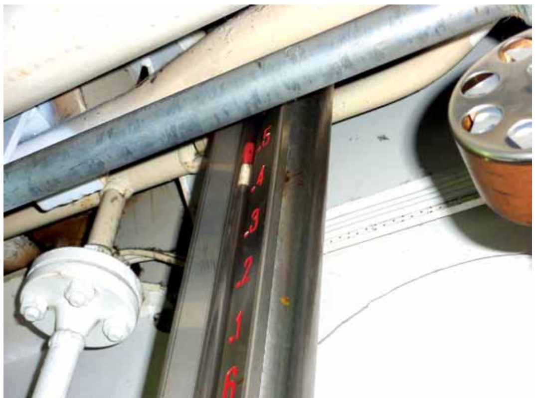
^ Bunker tank level indication
