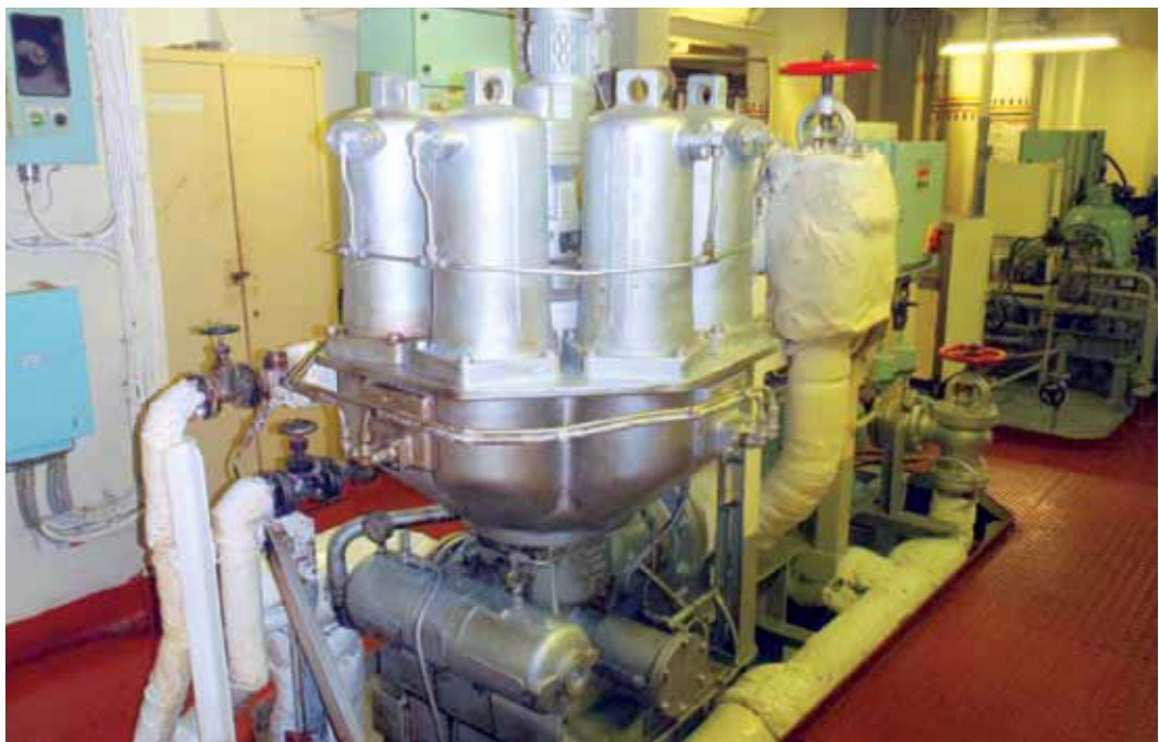
^ Fuel oil filters
