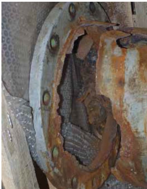
^ In service failed pipe
