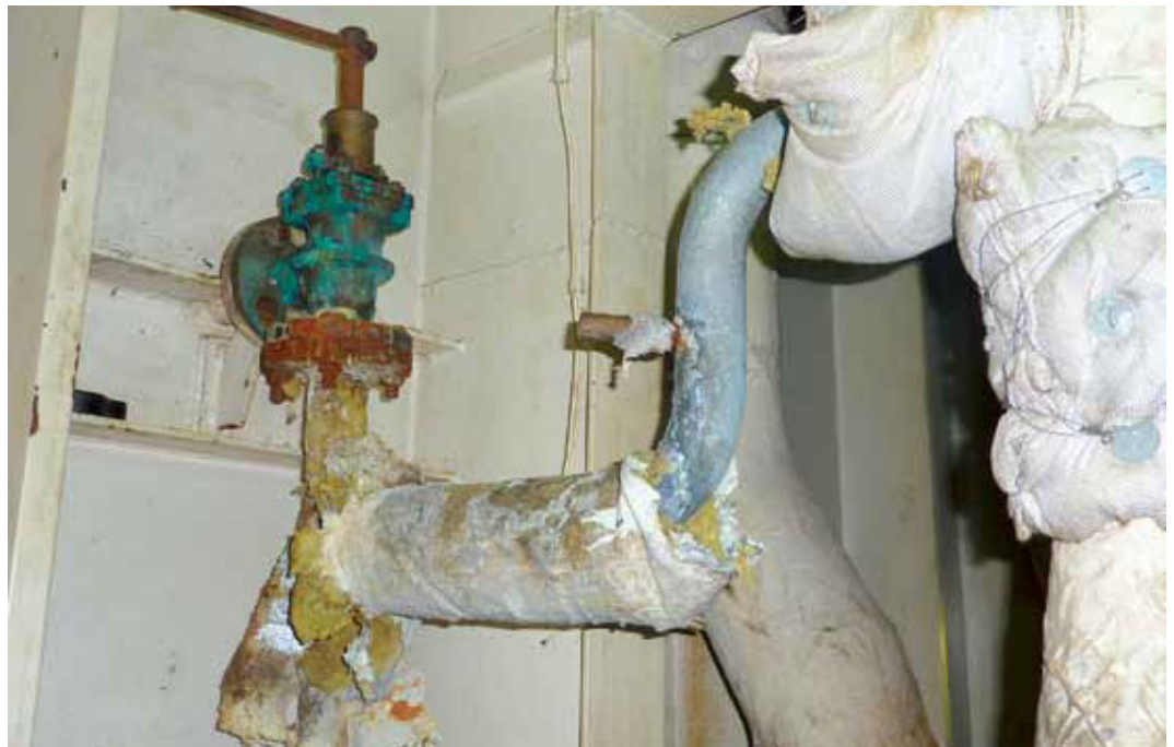
^ Temporary wooden plug in steam line, which is HIGHLY DANGEROUS
