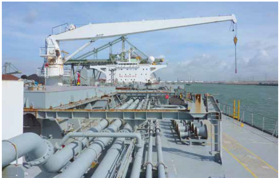
^ Typical cargo piping
