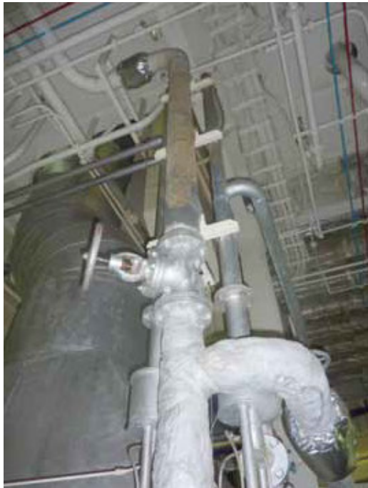
^ Typical steam piping
