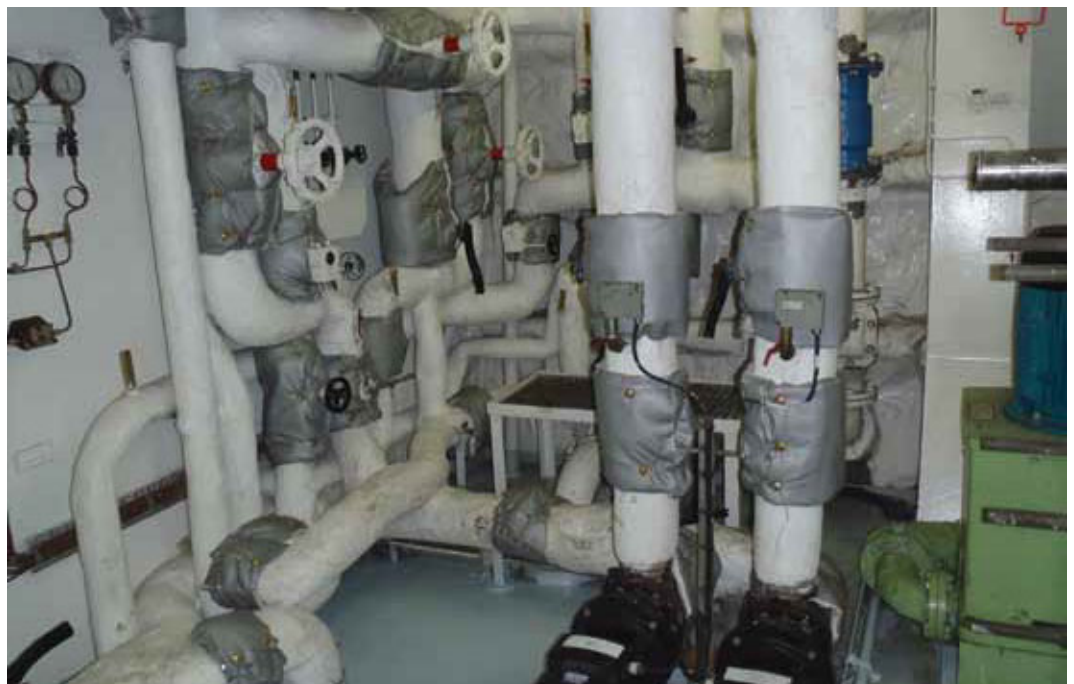
^ Typical thermal oil piping
