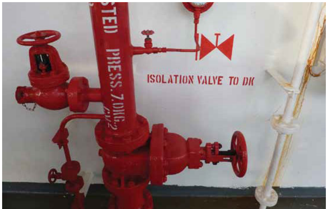
^ Typical fire main piping
