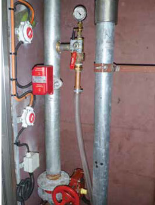
^ Typical sprinkler system piping
