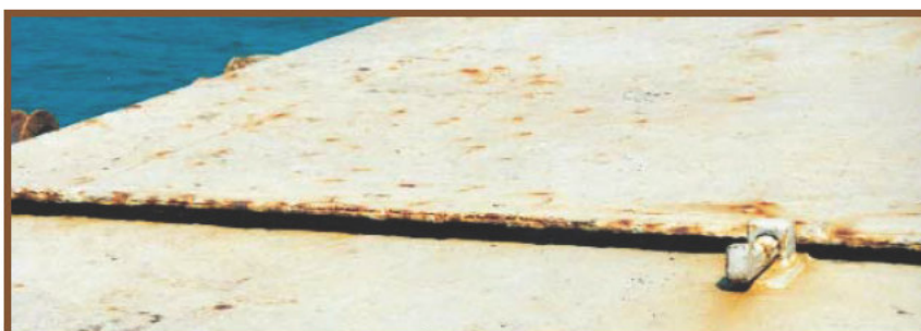
Two panels shown out of alignment.
