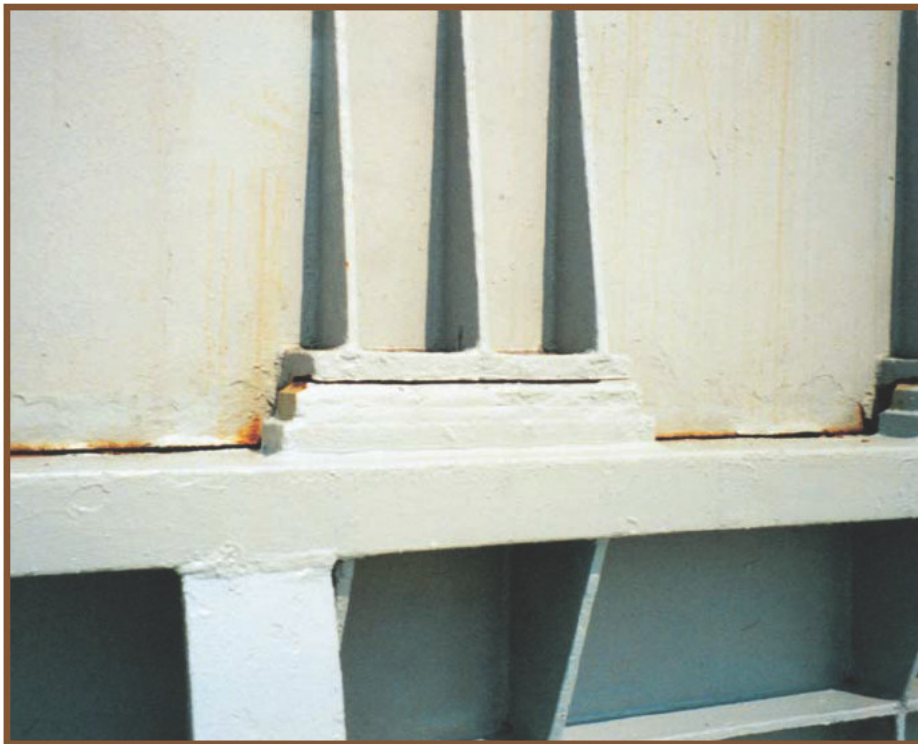
Worn 'steel-to-steel' contact points.
