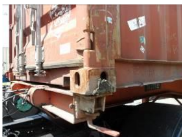
Figure 6.2 Mud in corner fitting
